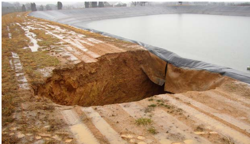
2003 Sinkhole on the berm of the impoundment
